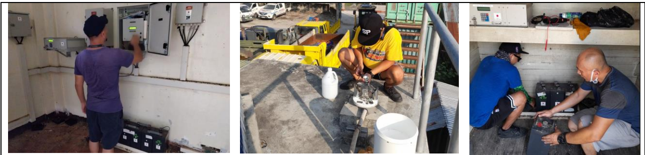
Above pictures show some of the activities carried-out during Quarterly Maintenance by the PRBFFWC: (top left) Checking & testing the overall telemetry system and communications; (top middle) Cleaning and testing of rain gages; (top right) checking of all other station-related appurtenances such as solar cell batteries, etc.
