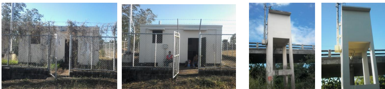
Above, the Sapang Buho RR-WL telemetry station before (L) and after (R) repainting and clearing activities.
