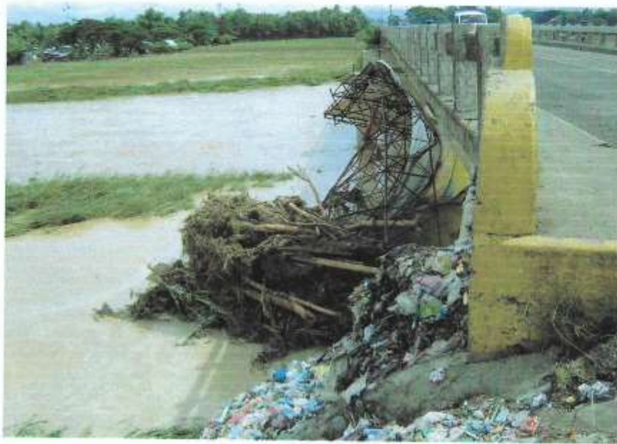
Pic 1.0 Debris brought by the flashflood caught under the Doña Josefa Bridge at Inang Bayan, Brgy. San Vicente, Gapan, Nueva Ecija.
