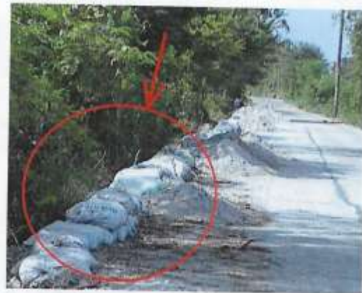
Pic 4.3 Sandbags protecting the Arayat-Cabiao Ring Levee at Bgy. Sta. Cruz, Arayat, Pampanga during the event.
