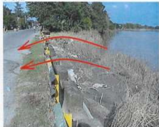
Pic 26.10 A section along the municipal road in Bgy. Pasig, Candaba where Pampanga River overflowed.
