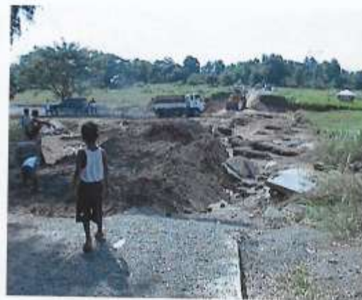
Pic 6.3 Breached road dike going to Sitio Kaingin in Bgy. Sumacab Norte, Cabanatuan, N.E.
