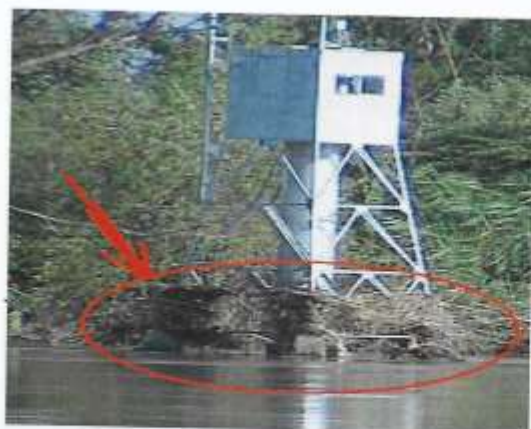
Pic 9.2 Dried branches and debris clinging to the foundation of Zaragoza telemetering station after the flood event.
