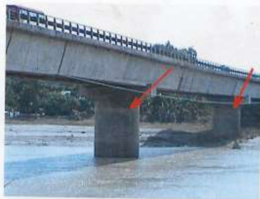
Pic 20.0 High water marks at the bridge's post of San Agustin Bridge in Arayat, Pampanga.
