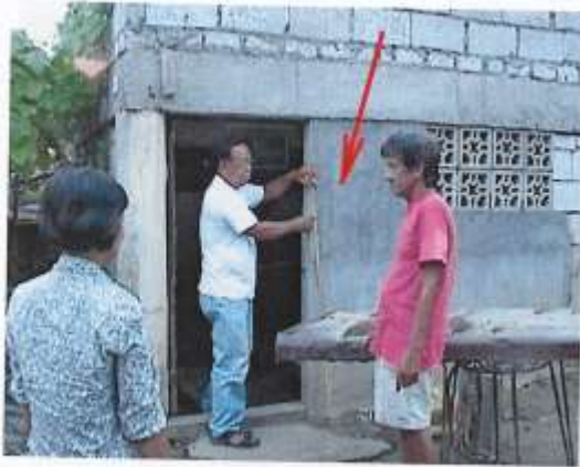
Pic. 21.0 Maximum flood height reached 1.3 m in Bgy. Sta. Monica, San Luis, Pampanga. (peaked on August 29, 2004)
