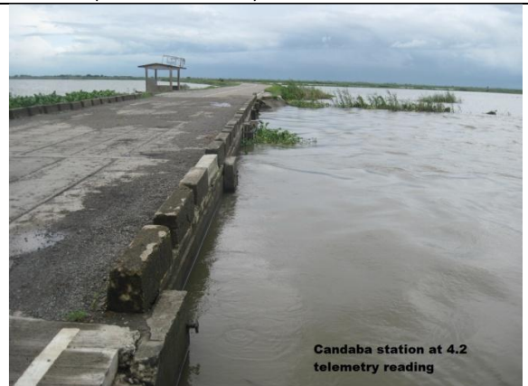
The bridge adjacent to the Candaba station at 4.20 meters' telemetry reading. Note that at around 5.0 meters water is almost above the bridge's floor
