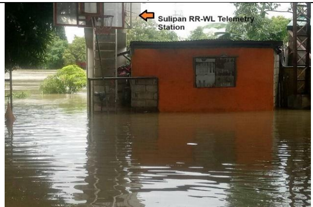
The Sulipan RR-WL telemetry station which was already surrounded by floodwaters at around 1300H of July 31, 2023, TC Egay-Falcon event (photo taken by Ms. W. Flores)
