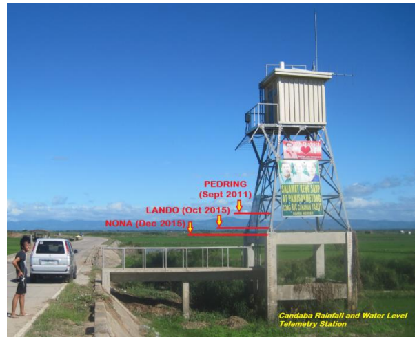
A view of the station with various flood level peaks attained during 3 different events from highest to lowest level – Pedring (Oct. 2013), Lando (Oct. 2015) and Nona (Dec. 2015)
